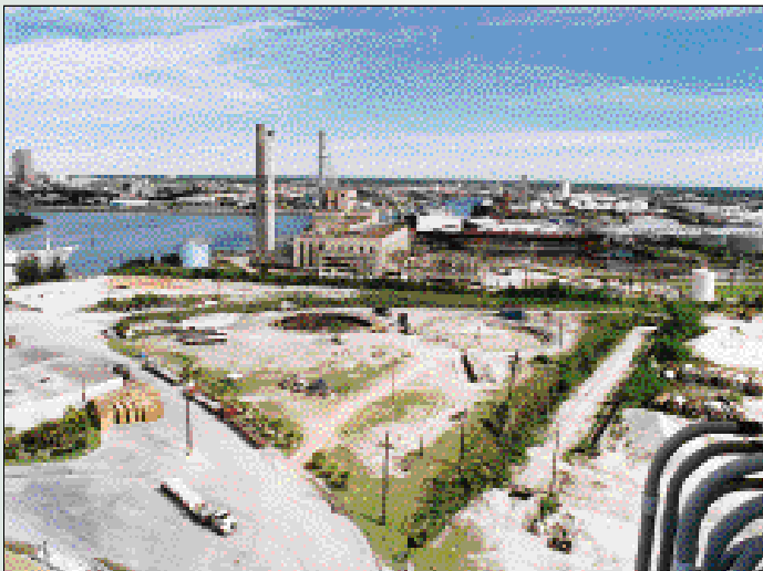
At this former site of a cement manufacturing facility in Port of Tampa, Fla., Brown and Caldwell excavated 12,000 tons of contaminated material from above-ground storage tanks. The use of risk-based cleanup levels—the first in the state—sped completion of the cleanup and meant that more than 24,000 tons of soil could be used as backfill or left in place.
